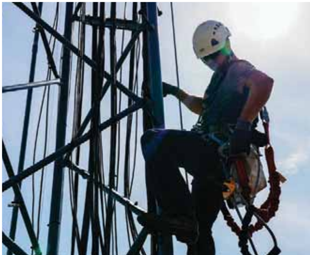
Internet Service Technician Mike McDade climbing one of the co-op's many wireless internet towers.
