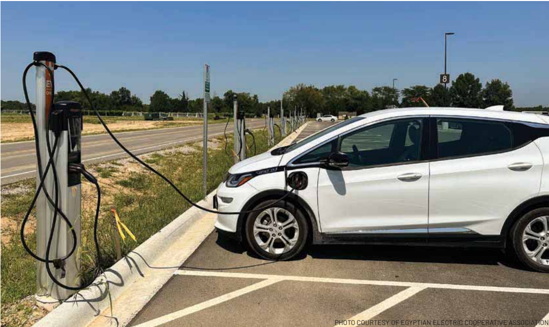
PHOTO COURTESY OF EGYPTIAN ELECTRIC COOPERATIVE ASSOCIATION
