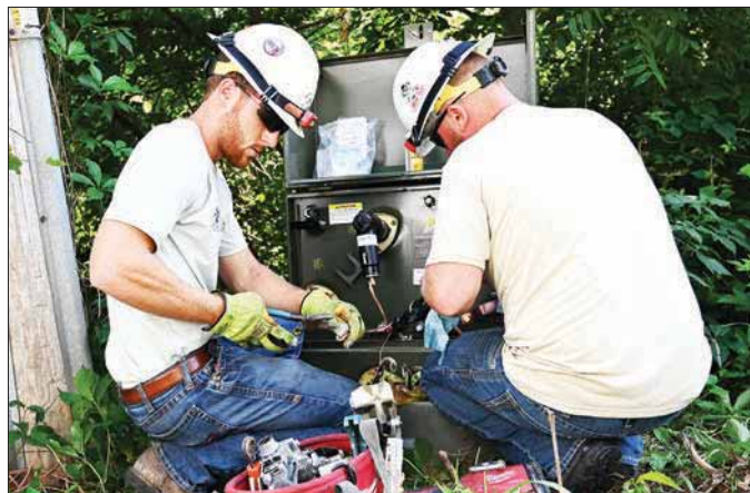
Above, Rock Energy workers access a padmount transformer at a residential home in one of the co-ops service areas.
