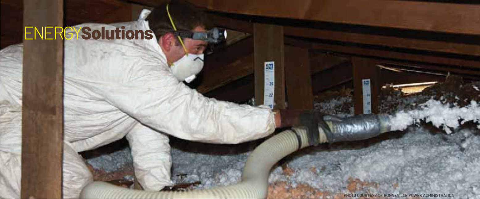
PHOTO COURTESY OF BONNEVILLE POWER ADMINISTRATION
