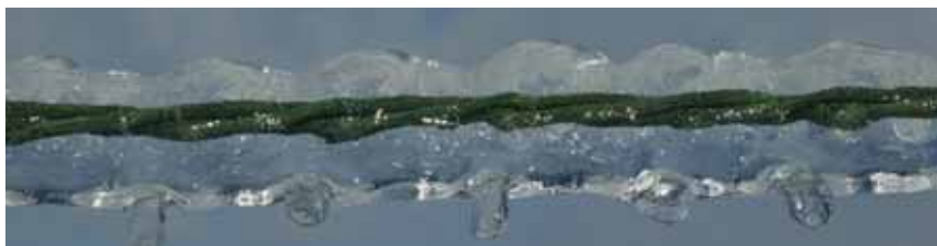
Utilities become concerned when ice builds up to a quarter inch or greater.
