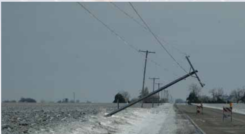
Ice buildup on power lines and poles, plus high winds, can cause galloping lines and poles to fall.
