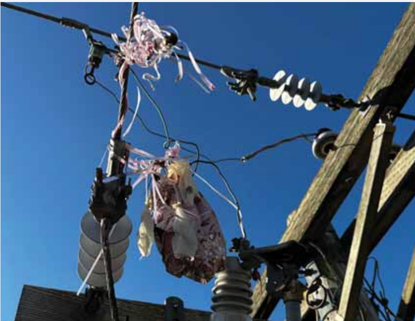
Lineman Matt Kish responded to an outage caused by mylar balloons that were entangled in the power lines on Nov. 18 off Levi Road.
