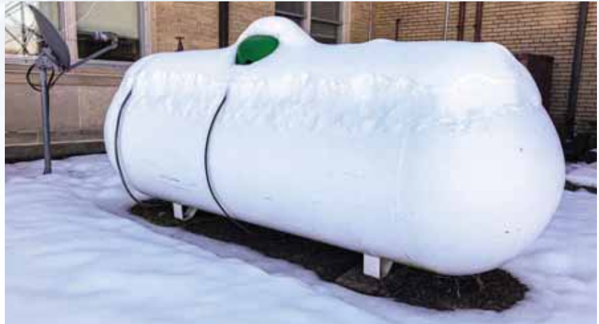
Keeping your propane tank free from snow and ice will allow your propane provider safe and easy access to service your tank.
