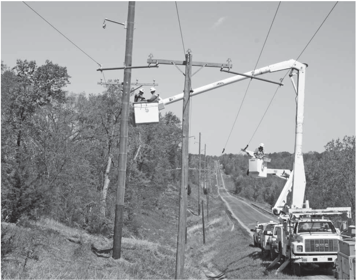
Work is underway on a new transmission line from Smithfield to Ipava. The line will connect two substations and will improve reliability of service for members.
