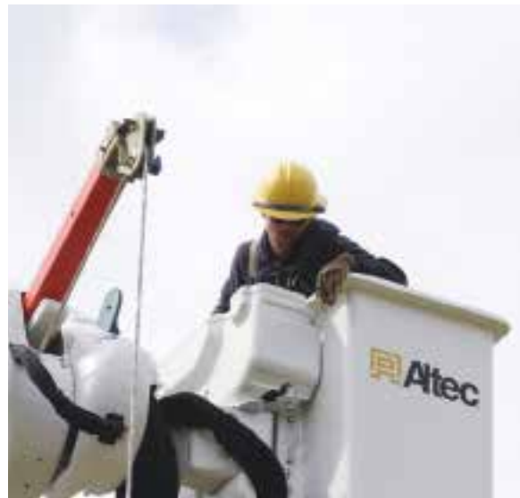
Linemen participated in the Bucket Truck Obstacle Course during Association of Illinois Electric Cooperative's 17th Lineman's Safety Rodeo held in Springfield, Ill.
