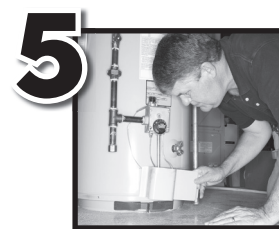
5 New water heater
