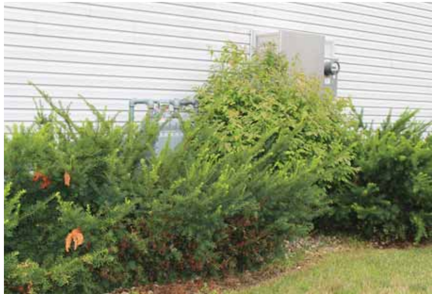
Shrubs prevent easy access to this gas and electric meter, making it difficult for co-op workers to read meters, do routine maintenance, and handle emergencies.
