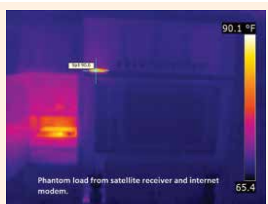
The infrared picture shows where hot spots are located; in this instance heat is coming off the satellite receiver and the Internet modem. This represents electricity in use or Phantom load.
