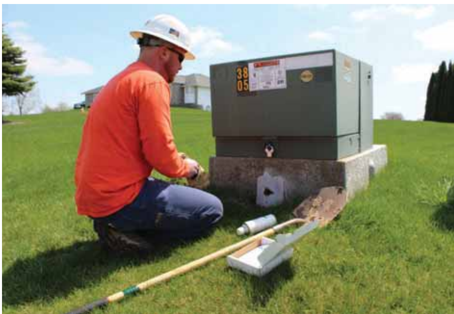
Lineman Bill Wright repairs a small hole in a pad-mount transformer on Nickolas Way in Rockton.
