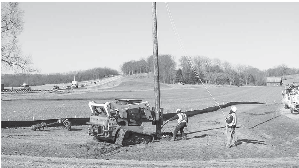
A skid loader is used in muddy conditions on Sister's Creek off Route 24 to set poles. Lineman Donnie Schrodt (L) is making sure the pole is in the right spot to set it, while Lineman Rick Roudebush (R) is lining up the pole for proper placement.
