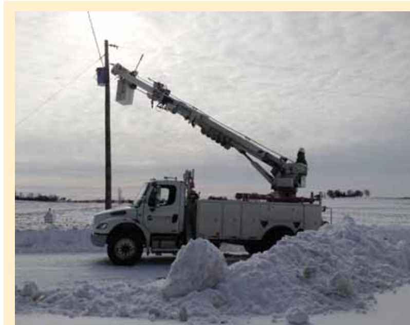
Shelby Electric Cooperative foreman Brian Chevalier (in bucket) and line-man Jamie Sharp work on restoring power to approximately 600 members who were without power following an early January winter storm.
