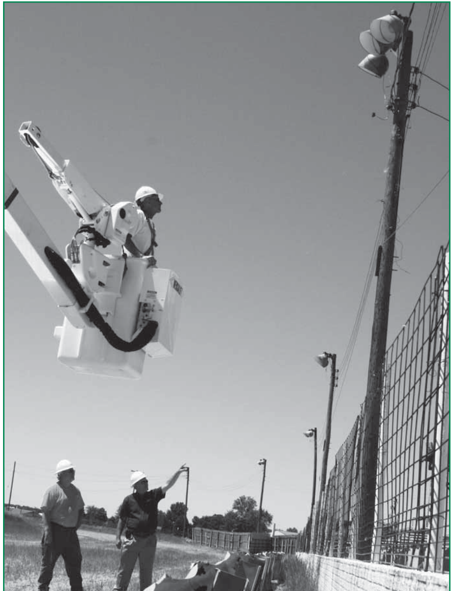
Spoon River Electric Cooperative Lineman Donnie Schrodt (in bucket truck), Manager of Operations Frank Romane (left) and President/CEO Bill Dodds discuss an electrical upgrade project underway at the Fulton County Fairgrounds in Lewistown. The project will provide safer, more reliable electricity at the fairgrounds.
