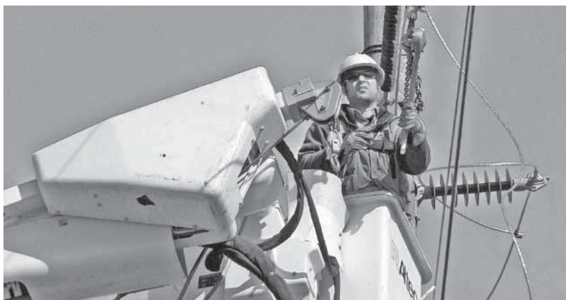
Steve Gottman of Prairie Power, Inc. works on line improvements. PPI is beginning a large upgrade of lines and equipment on Spoon River Electric Cooperative lines between Ipava and Knoxville.
