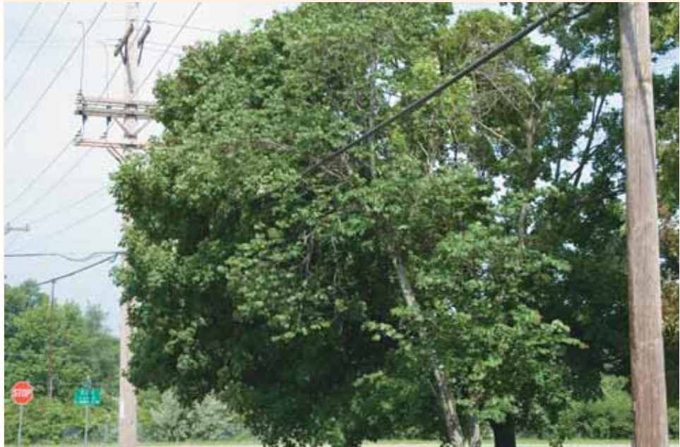
National standards for electrical safety require that branches within 15 feet of electrical equipment be removed. Be careful when trimming tree branches near power lines. If a tree presents a safety concern call the cooperative for help.
