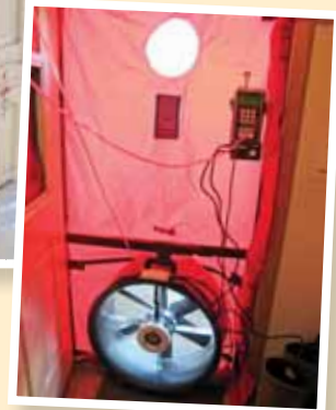
Below: Blower door apparatus used to simulate wind hitting the house from all sides to help expose air infiltration.
