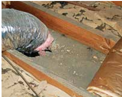
This photo was taken in the home of Marla Eversole. Note the way the insulation is rolled away from ducting, leaving no insulation in that area!
