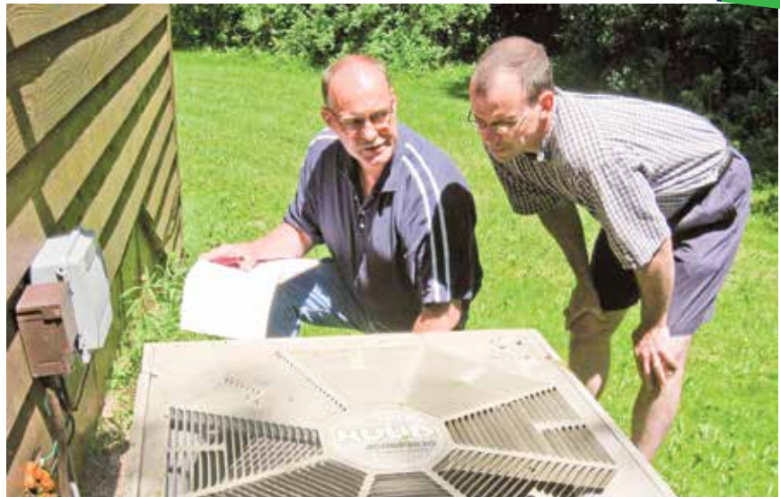
Energy assessor Dale Oas, left, recommends that Brian D’Haeze replace his home’s central air conditioning unit with a new, energy-efficient model.
