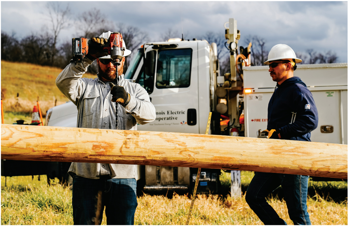
Journeyman Lineman Josh Davis and Apprentice Lineman Kaiden Davis working on a pole replacement in Pike County.
