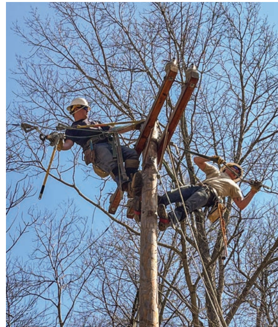
Journeyman Lineman Jake Keys (right) and Apprentice Lineman Carter Hays (left) repair damage after a recent wind and rain storm
