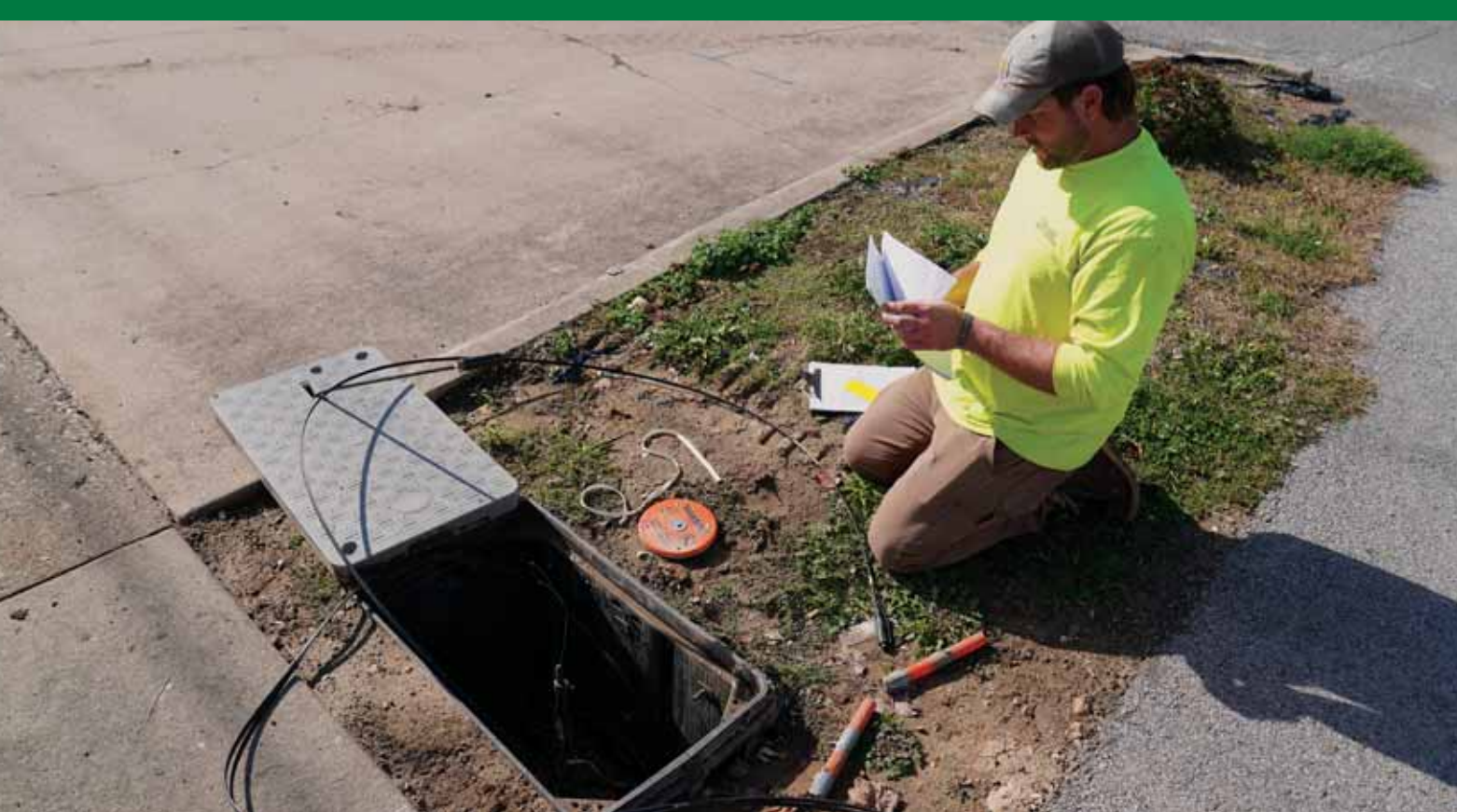
A crew member with Wiemelt Excavating finishing up a fiber drop in Hardin.
