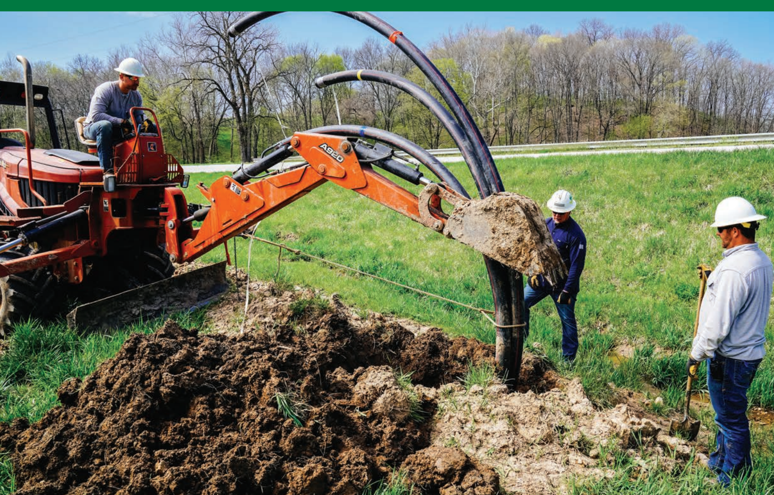
Apprentice Lineman Kaiden Davis, Line Foreman Brad Kemper, and Journeyman Lineman Josh Davis working on an underground line near Barry.
