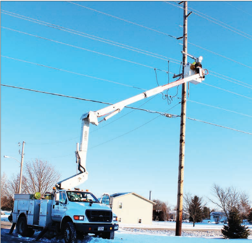
Pictured above, a Rock Energy crew works on a power line following a winter storm in Rockton, IL.
