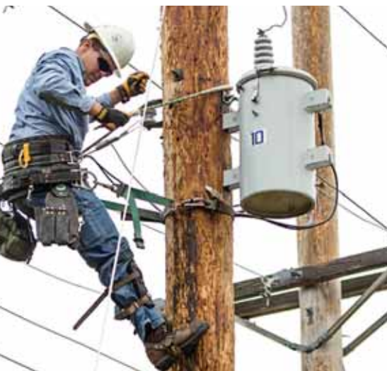
Apprentice Lineman Justin Hubert is doing his part in the H-Structure Obstacle Course.
