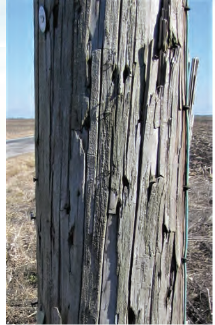
Deterioration of outer shell
