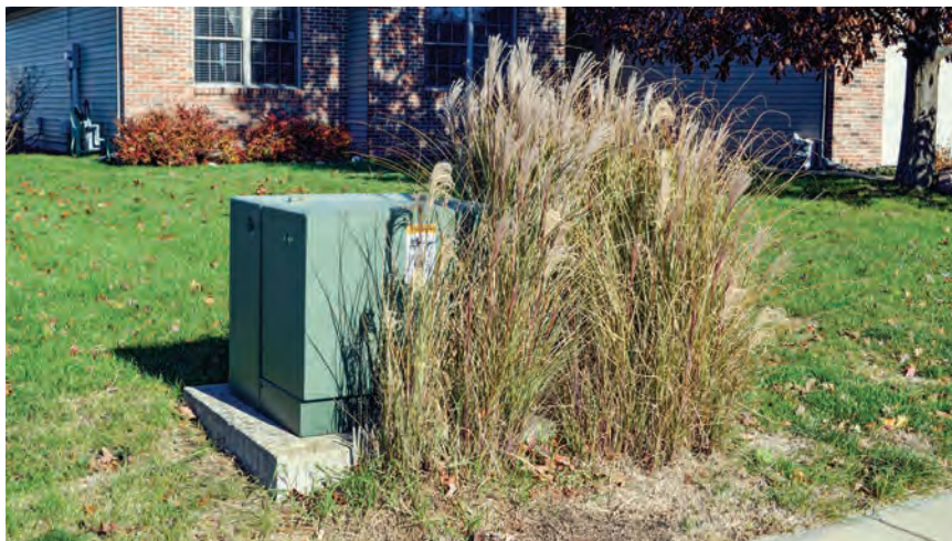
Do not plant shrubs close to padmount transformers or other utility equipment. We need at least 10 feet of clearance in front of the transformer.
