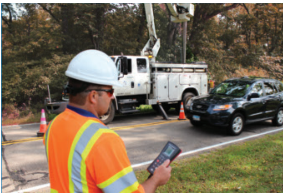
Pictured above, Rock Energy Operations Manager Tony Haffelder monitors a work zone on Highway 67 in Clinton, WI.
