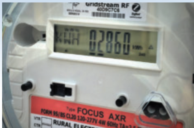
Meter displaying kWh consumption
