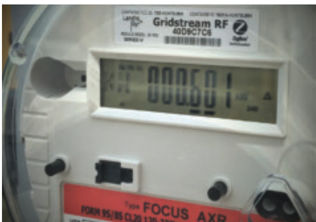
Meter displaying kW demand
