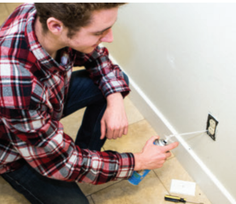
Electrical outlets on outside walls are a common source of air leaks and are easily patched. Photo: Marcela Gara, Resource Media
