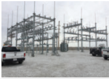
New Elvaston Substation
