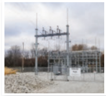
New Carthage Substation
