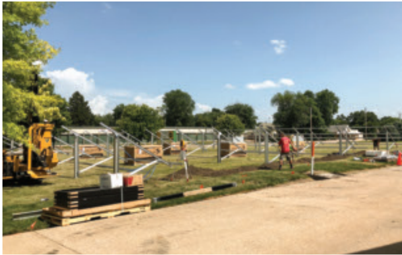
Eagle Point Solar construction crew assembling the Spoon River Electric solar array.
