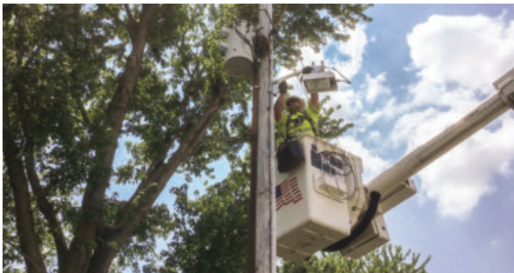
CCEC Apprentice Lineman John Schroeder installing a router on our pole as part of the AMI project.
