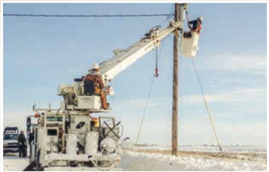
Even though linemen can still be found climbing poles, over the years, hydraulics and bucket trucks improved the safety and efficiency in building out and maintaining the cooperative's distribution system.
