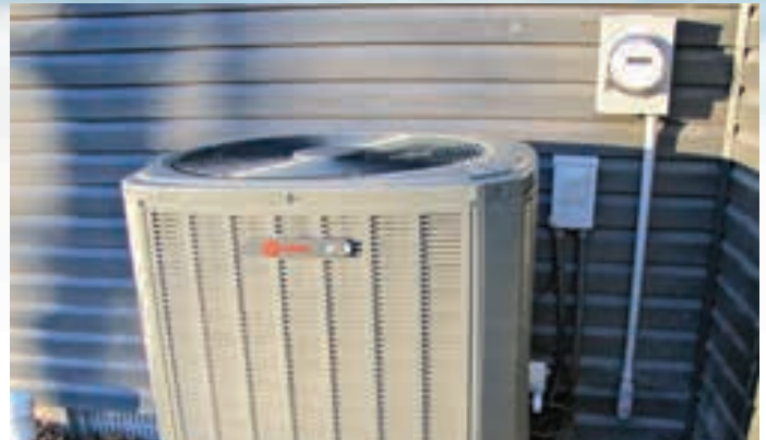
Dual Meter installed next to Trane heat pump
