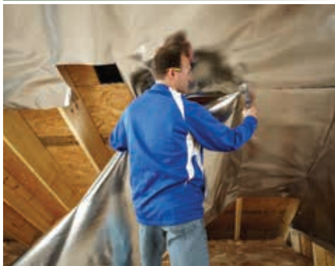
Foil is placed under the framing supporting the roof, reflecting unwanted radiant heat upward and out of the home. Photo Credit: Reflective Insulation Manufacturers Association International
