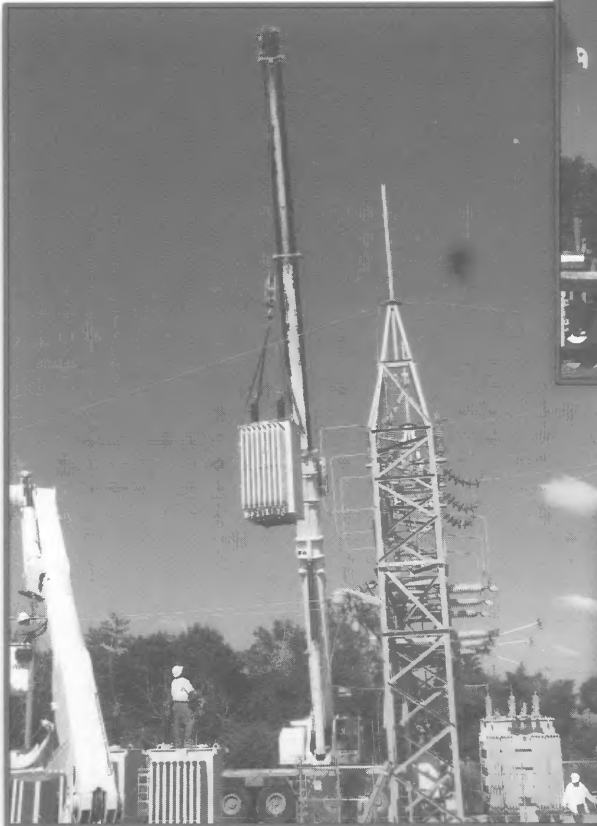
▲ Lifting out the old transformers was a big job. Here is one of the three smaller transformers replaced by the new, 33 percent larger, transformer.
