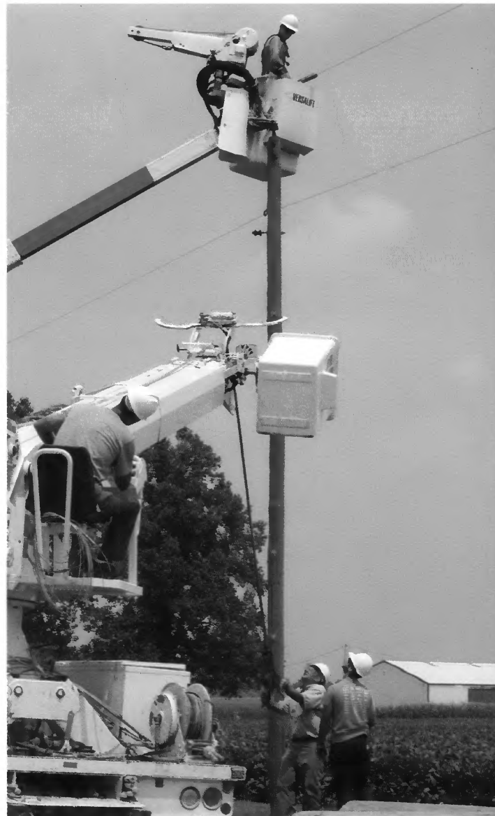
The old pole is taken down by Baird (in the bucket truck), Vedder holding the single phase line, and at the bottom of the pole, Dave Gant, area serviceman, and Cole Hurrelbrink, a summer college worker.
