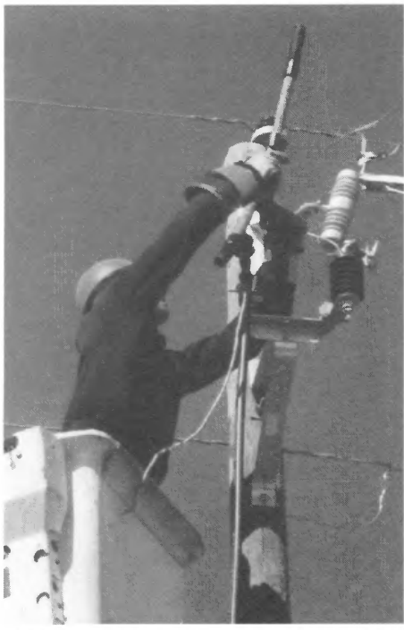
This lineman is trying to restore power. Improper generator use puts his life in danger.
