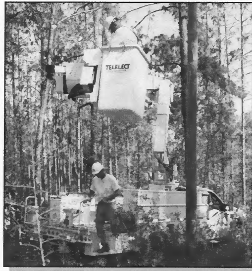
Damage in Mississippi caused by Hurricane Katrina
