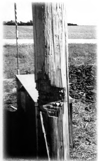
Vandalism has been known to create outages on cooperative lines.
