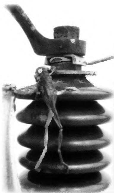
Last year, this frog caused an outage at EnerStar when it climbed across a transformer.
