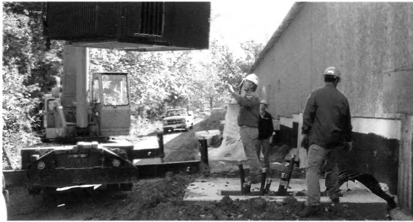
Northern Region employees install a transformer for underground service at Grand Bear Lodge in Utica.
