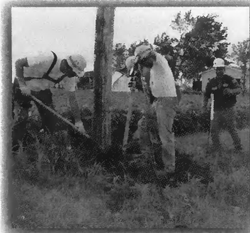
Journeyman Lineman Ryan Campbell, Maintenance Foreman Scott Farmer, Journeyman Lineman Steve Rosenthal and Construction Foreman Richard Lingemann work together to change-out a pole in Galva after storms damaged it.
