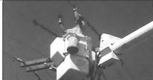
Once the wires were on the new cross arms, the wire was pulled to make sure it was taut. Hand signals were used to make sure they were positioned correctly.
