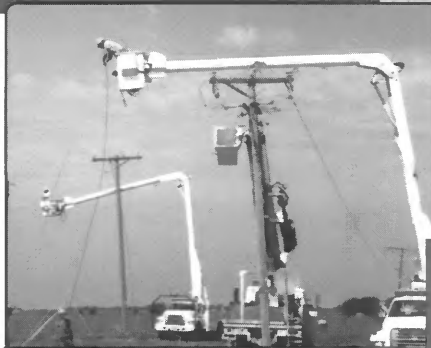
New wires were strung for the East-West line that crosses the highway. As the new wires were being strung, the existing North-South line, already taken off line until the work day was complete, kept the new wires from resting on the pavement.
