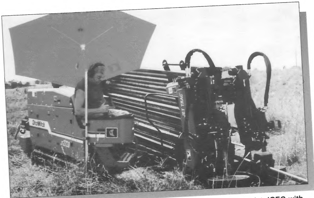
Petitgout Brothers, Inc. use a directional drilling machine to assist JCEC with cable replacement.
