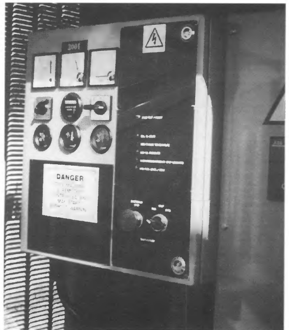
Control Panel on the 125 KW GENSET
