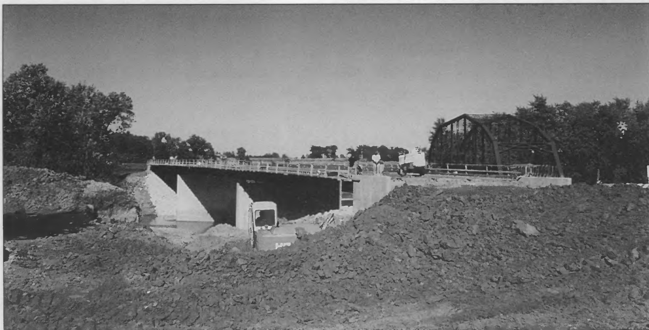
The department oversees construction of new bridges like this one, which will replace the short, narrow span in the background.
