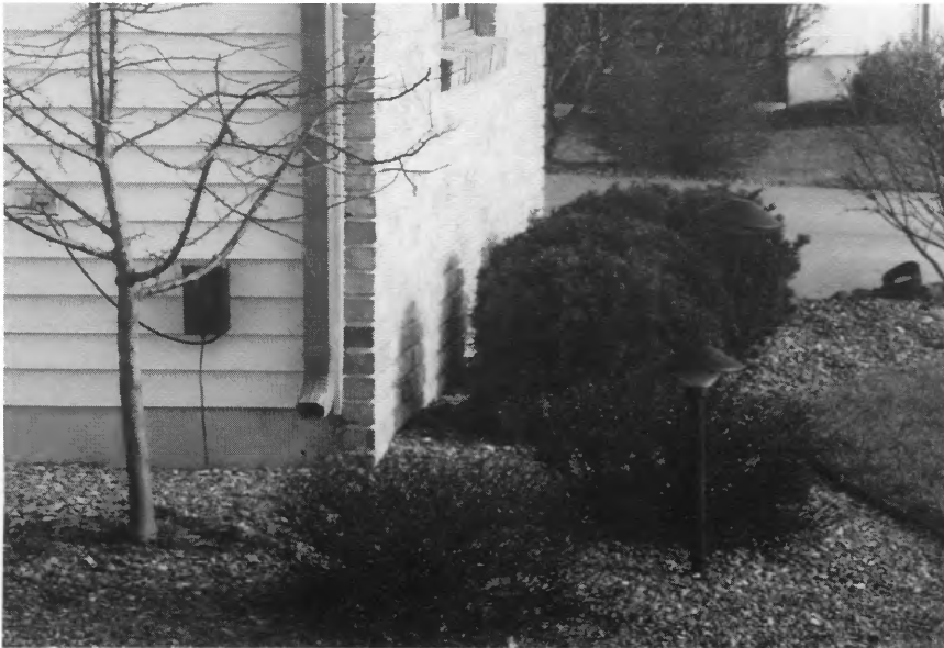
A fairly typical low-voltage lighting installation is pictured here. While not all the lamps are visible, the transformer unit and exterior wall outlet are. This installation is simplified because the wire is concealed under the decorative gravel rather than being in a trench. Note the mix of spotlights and floodlights.
